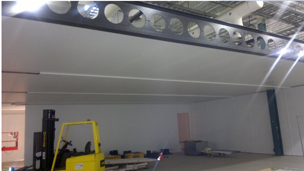
Ceilings supported in the web of the steels (shown) or on top of the steels
